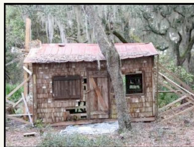
Cabin with straightened chimney .
